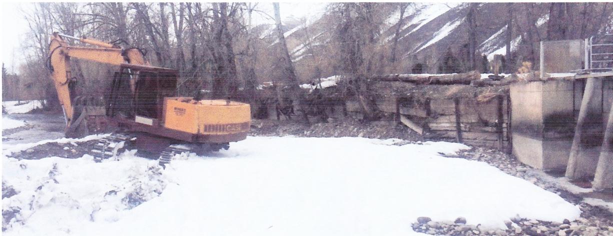
April 2 Removing the gravel bar that is keeping the rising river from reaching the Main gates.
