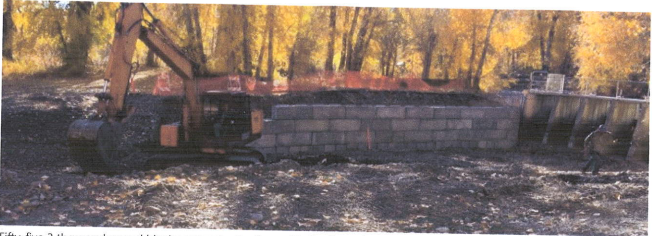
Fifty-five 3 thousand pound blocks set up to stay for awhile in place of the 60 year old boards that were in final stages of usefulness.
